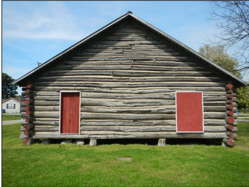
Figure 1-12. NRHP-listed American Legion Post No. 72 (CY0071) in Knobel, rear façade, view southwest (DSCN 1631).
