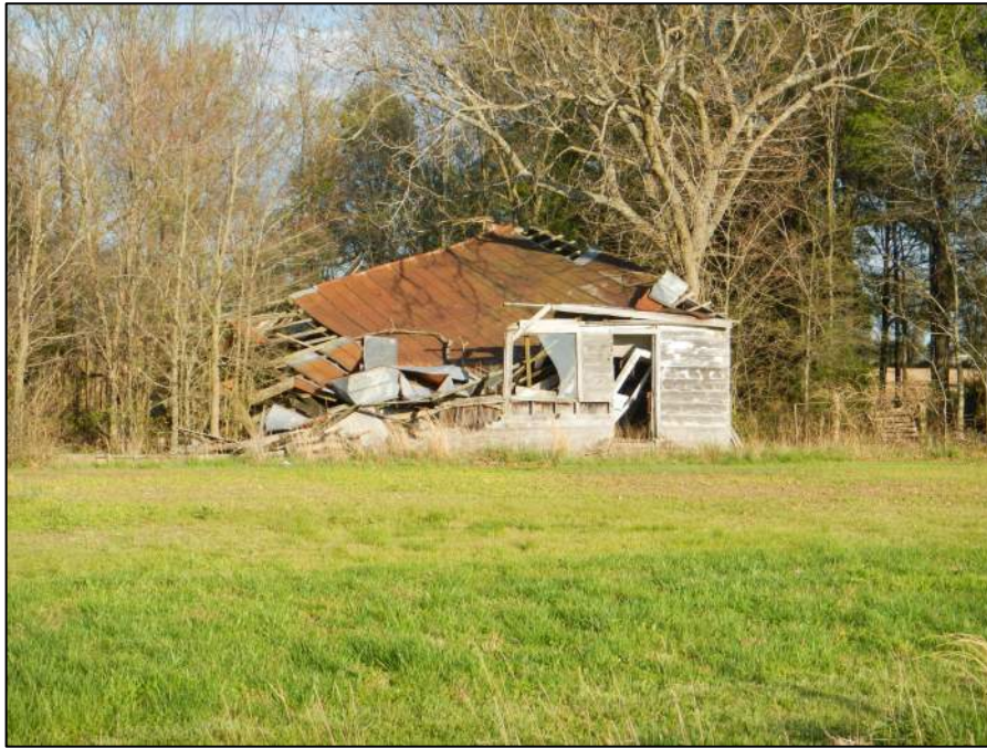
Figure 2-68. Property 15, collapsed south structure, view east (DCNS1805).
